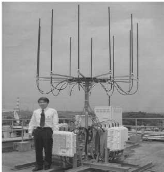
Example of Practical antenna and base station units
